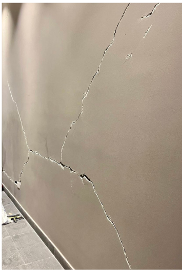
Damage to our hotel in Ibagué, Colombia, from the recent 7.4 earthquake.
